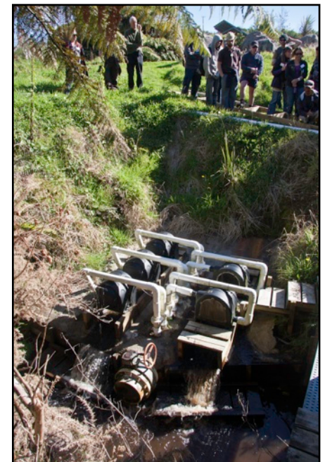
Above: Microhydro turbines turn the waters of the creek into electrical energy.
