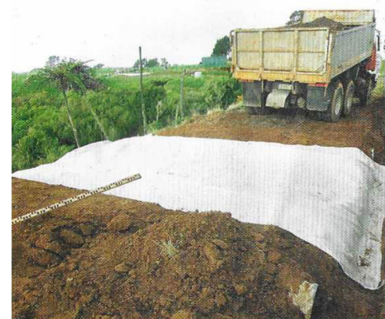
Filter fabric being installed on a 'reverse speed hump' on Daniel and Bena's driveway. Photo: GreenBridge.co.nz
